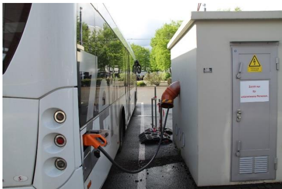
Fig. 1. An example of a plug-in charging system (Bremen)
