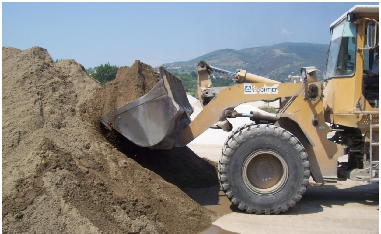
Fig. 5. Testing of a Z-kinematic loader in Skopje Cement industry “Titan” -Usje (Photo:J. Jančevski)
