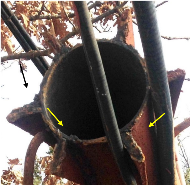
Fig. 4. The critical section at the welded joint
