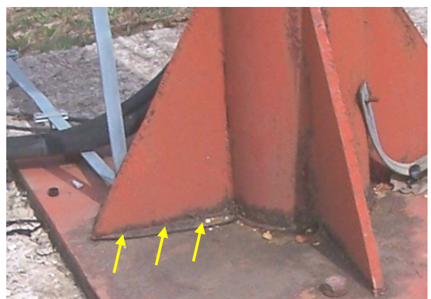
Fig. 7. Tensile crack caused by corrosion
