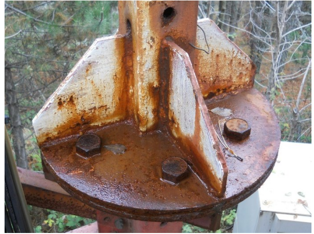
Fig. 5. Corrosion of the connecting flange
