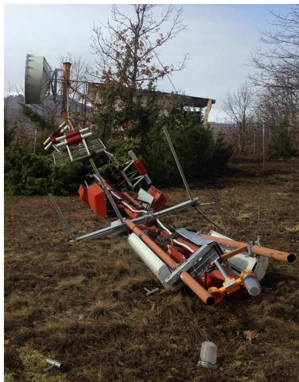
Fig. 3. Photo of the fallen mast segments
