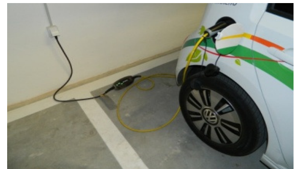
Fig. 4. Charging socket at EV
