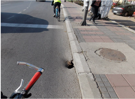
Fig. 5. Damage along the roadside
