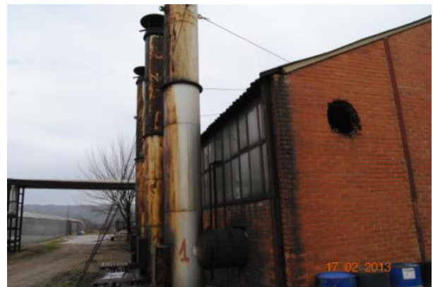
Fig. 5. Boiler chamber with chimneys
