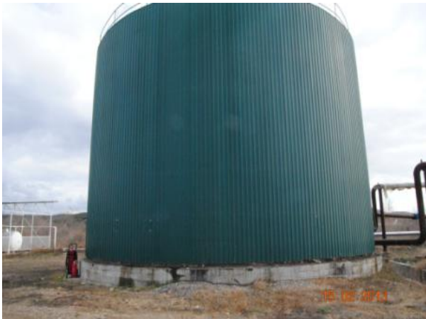
Fig. 7: Hot water reservoir. Capacity: 50 t. temperature: 65°C
