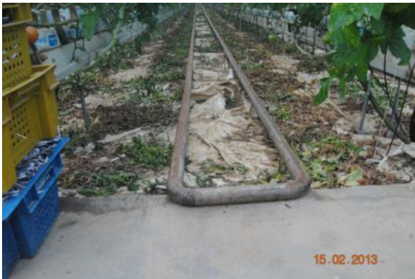
Fig. 2. Heating pipes. Material. Black steel. Purpose: The heating pipes are also used for movement of the harvesting carts
