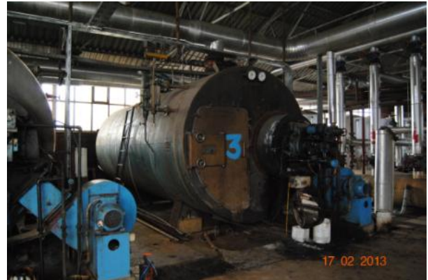
Fig. 4. Heavy oil boiler. Installed in 1973; heating capacity: 6 ha; place of origin: The Netherlands
