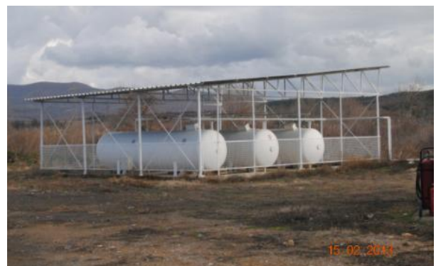
Fig. 6. Propane-butane tanks. Usage: Installed but not in function
