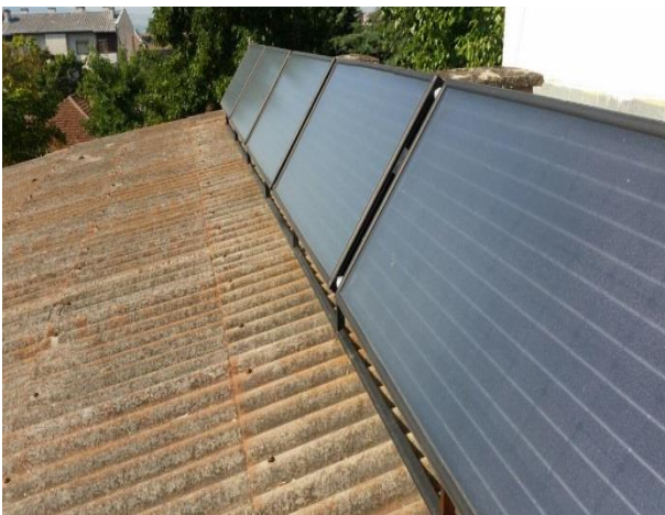
Fig. 1. Installed hybrid (PV/T) system in the kindergarten „Pavlina Veljanova” – Kočani
